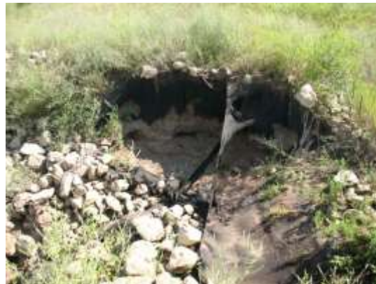
Photo 9. Blowout caused by rushing water from inlet pipe on south side of stormwater pond.
