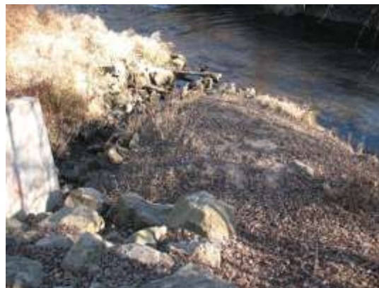
Photo 6. Stormwater inlet to river. The concrete structure is visible on the left.
