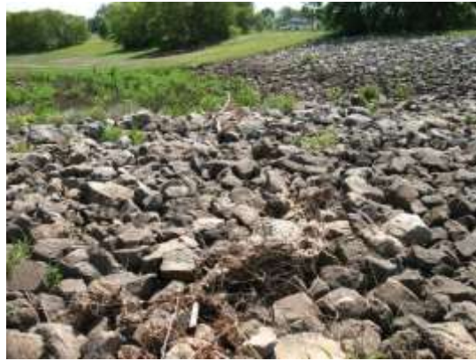
Photo 15. Extensive field of riprap on swale side-slopes at western end of park.
