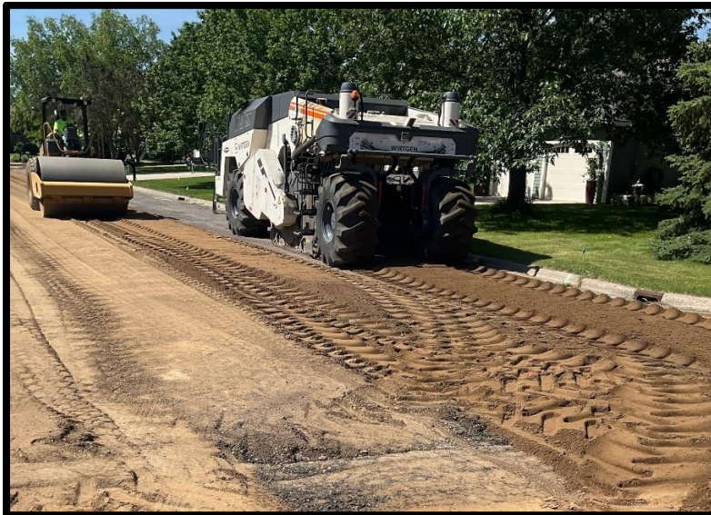
A reclaim machine was used to grind and mix existing asphalt with gravel base below A roller and road grader were then used to smooth out the gravel road
