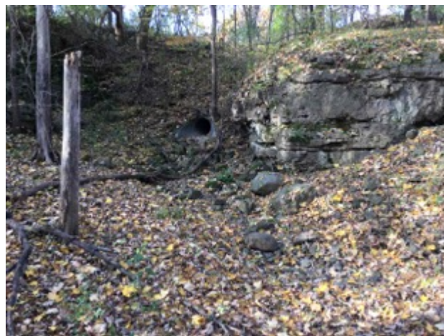
Photo 2. Culvert at west end of the gorge carries water during major rain events.
