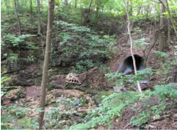
Photo 21. Culvert carries stormwater from south. Much trash and rubble has been dumped nearby. DF3.
