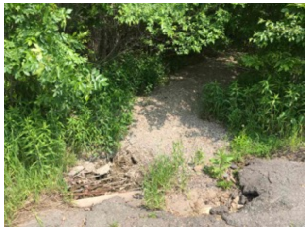
Photo 28. Culvert at the south end of the ditch that runs through DW2.
